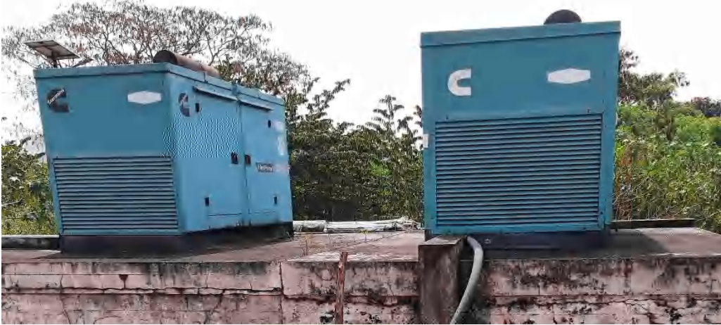
College Diesel Generator
