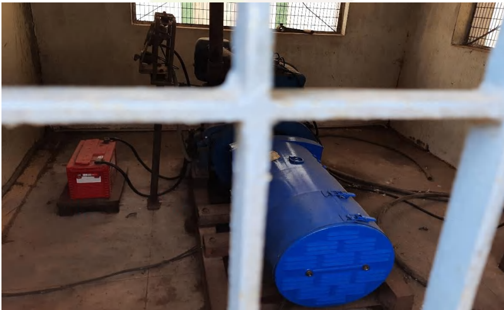
Hostel Diesel Generator
